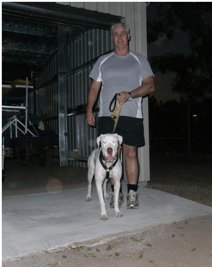
David Ewing and Flynn - concreter extraordinaire and helper, with their concreting handy work!
